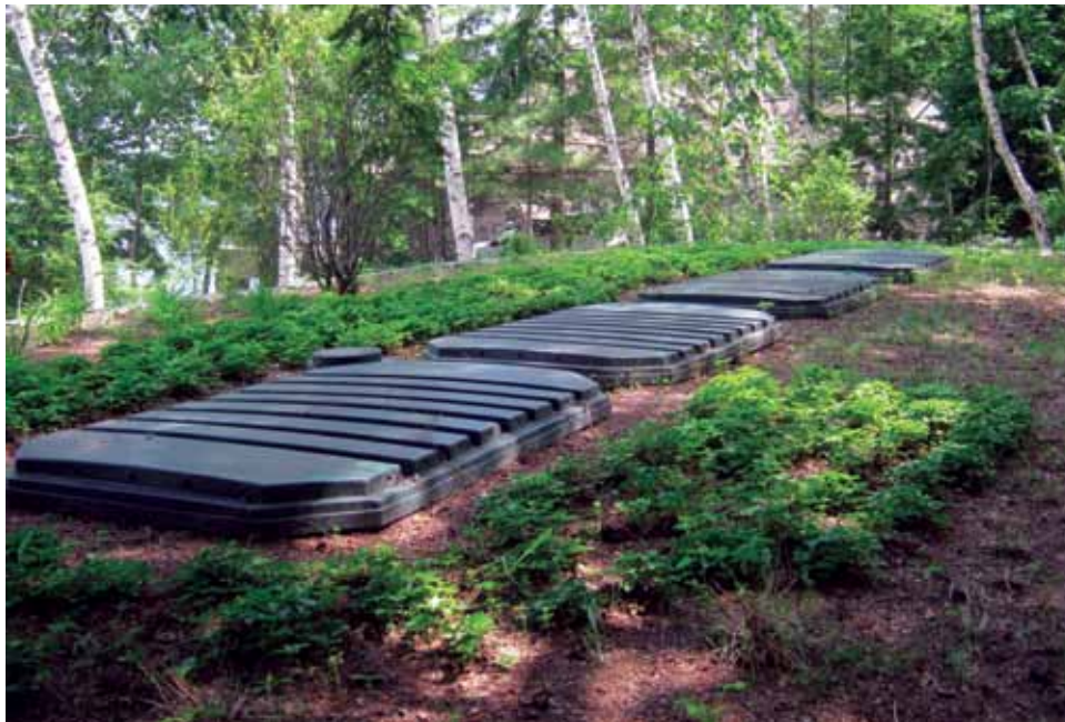
Native plants, an alternative peat septic system (shown above) and permeable pavers... all three combine at the Putnam's lake home ... creating a lake-friendly landscape to be envied!
